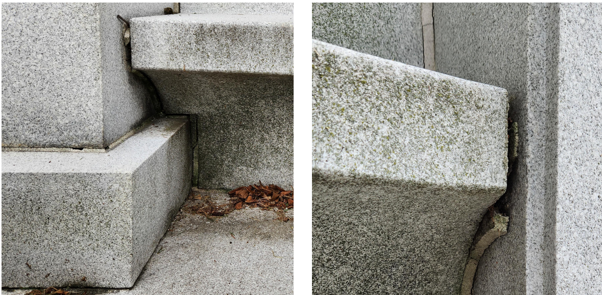
Figure 15. Deteriorating mortar and open joints at the east (left) and west (right) benches, Woolworth Mausoleum, 2023. Photos by author.
