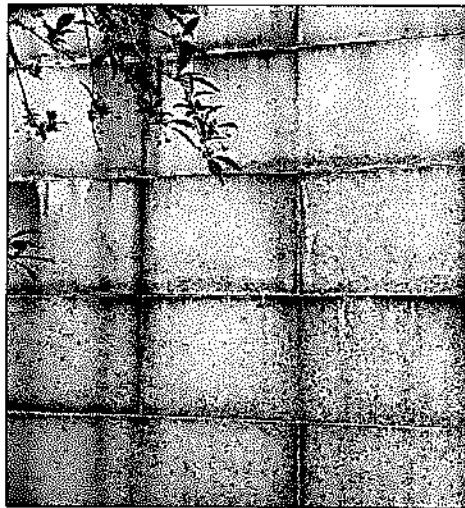
Figure 21. West-Facing Wall Damage
