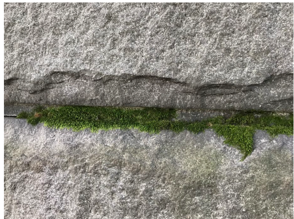
Figure 17: Moss growing in mortar joints
