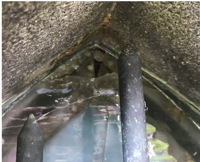
Figure 15: Broken glass, west window
