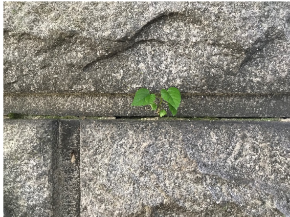
Figure 16: Disintegrating mortar pointing
