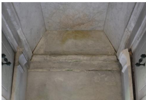
Figure 28: Water damage and salt damage
