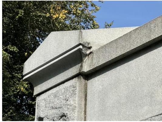
Figure 30: The mechanical damage
