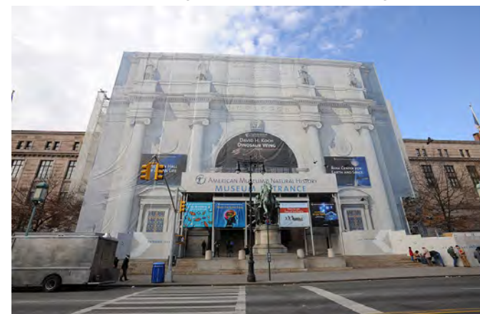
Printed scrim, such as one created for the American Museum of Natural History in New York City during a renovation, can be used to represent buildings around Main Street that have been lost.
