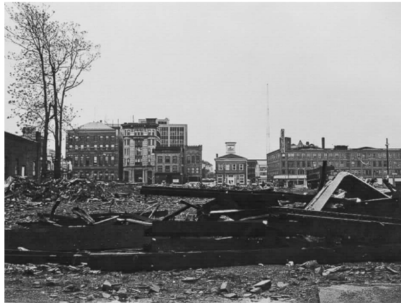
Demolition to make way for the construction of the new Civic Center. Old City Hall visible in the background.
