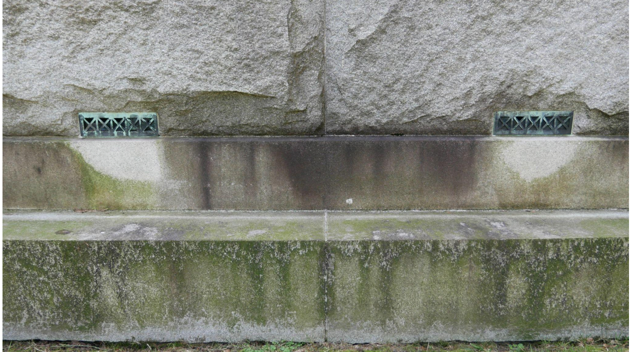
Image 11: Elizabeth Kostina, Gypsum and biological growth on Hickey Mausoleum's back side , 2024.
