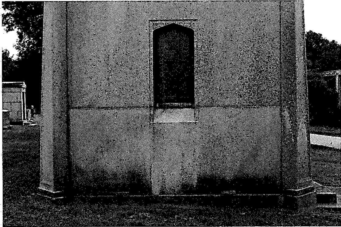
Image 6: The north elevation. Note the significant biological growth.
