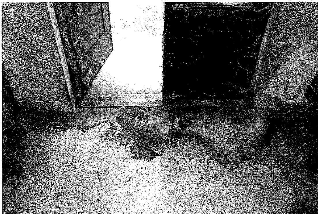
Image 7: Brown stains near door threshold, likely from water infiltration.
