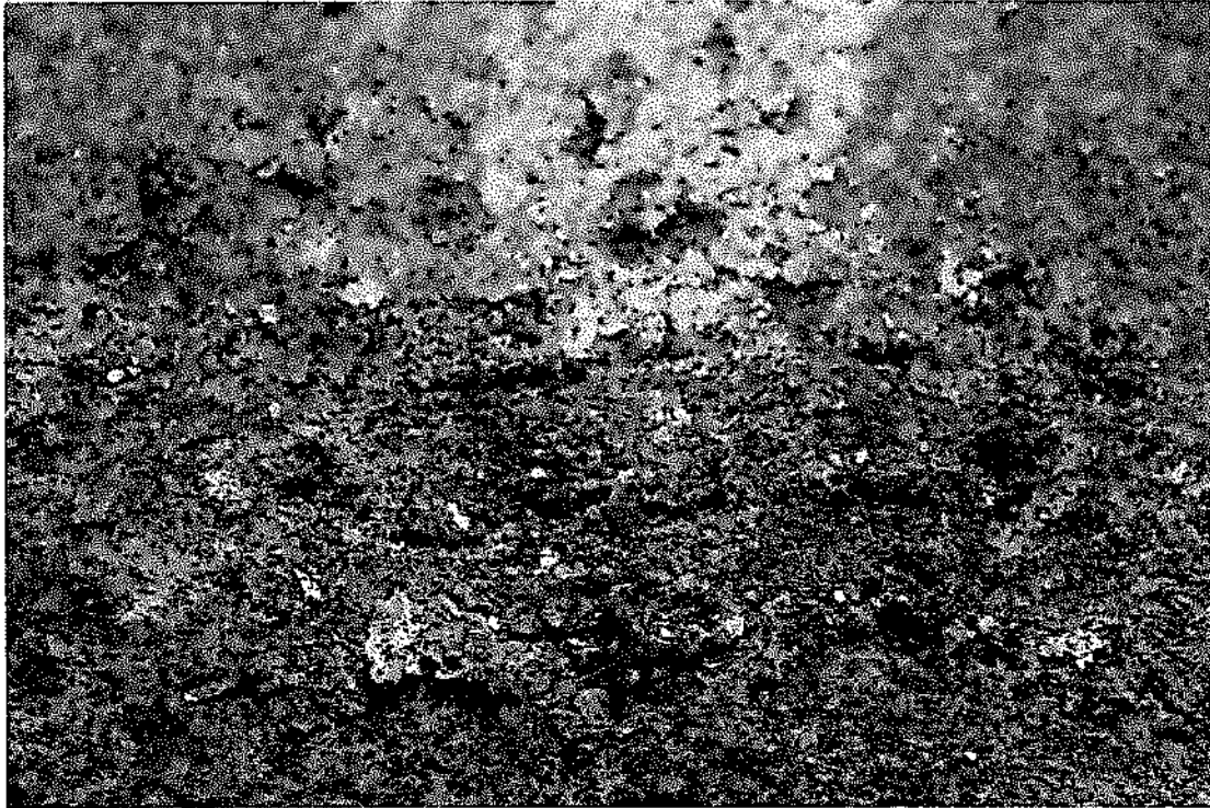
Image 8: Close up of the granite floor. Note the deterioration and flaking.
