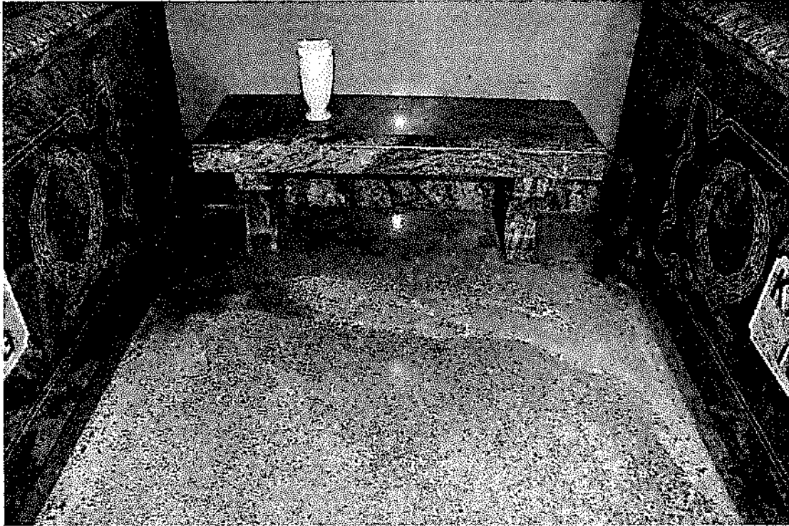
Image 10: Efflorescent staining on the floor.
