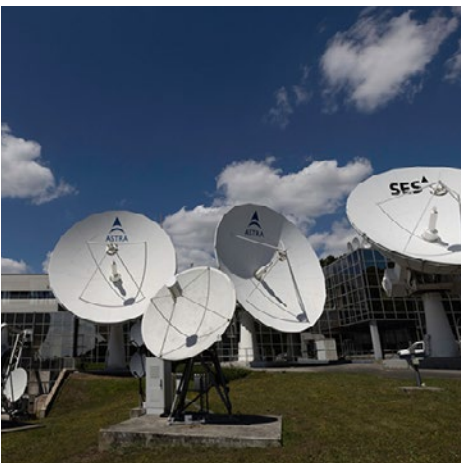
GOE-S satellite ground station
