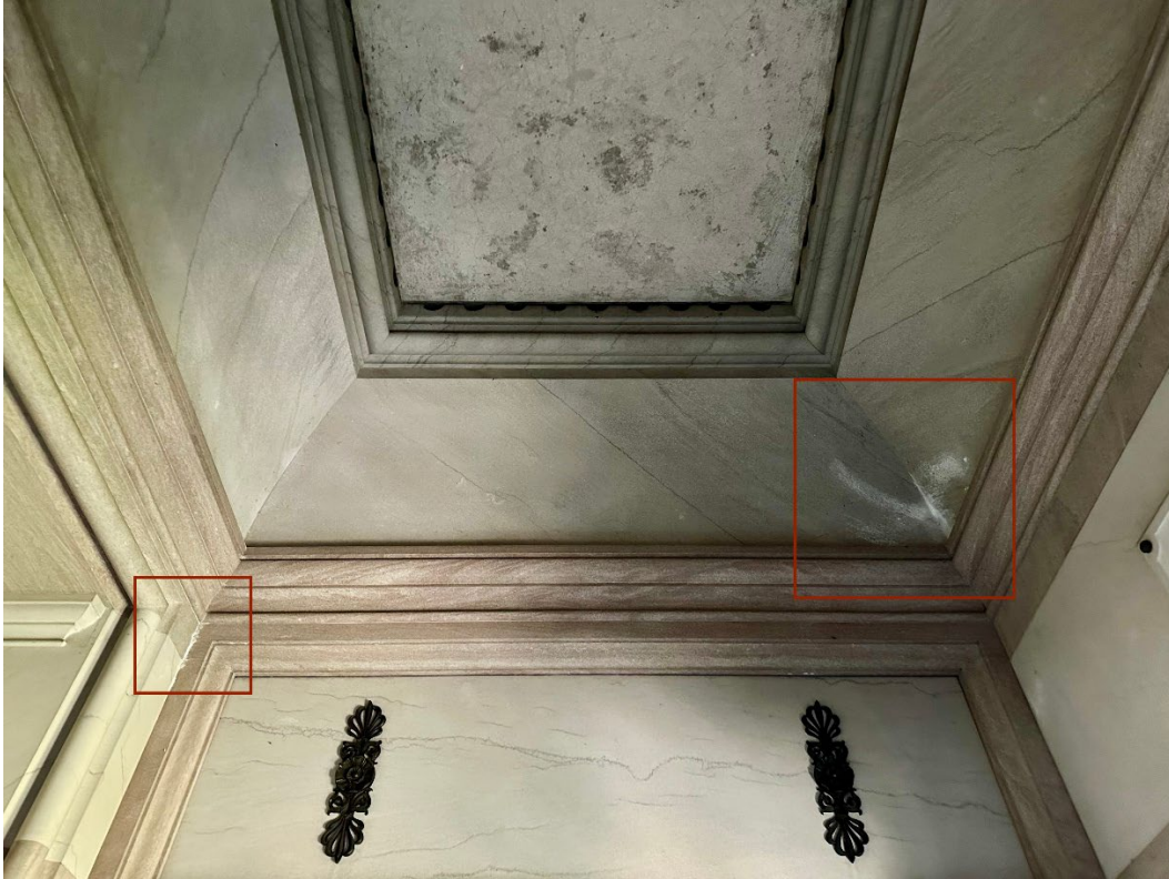
Figure 12: Yicheng Lin, Interior Efflorescent on the Corners , 2025.
