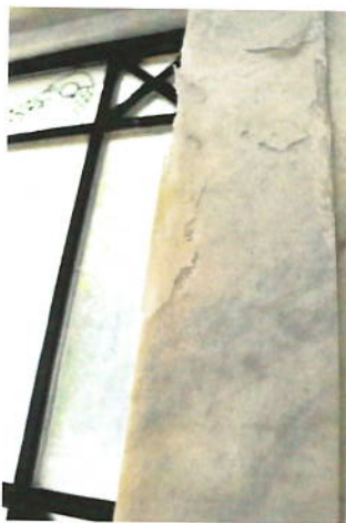
Figure 7 Deterioration of marble
