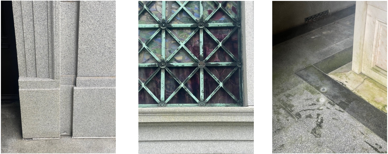
Figure 15: Mortar deterioration by entrance (Left), rosettes missing from exterior window grilles (Middle), biological deterioration on ground and tombstone (Left)
