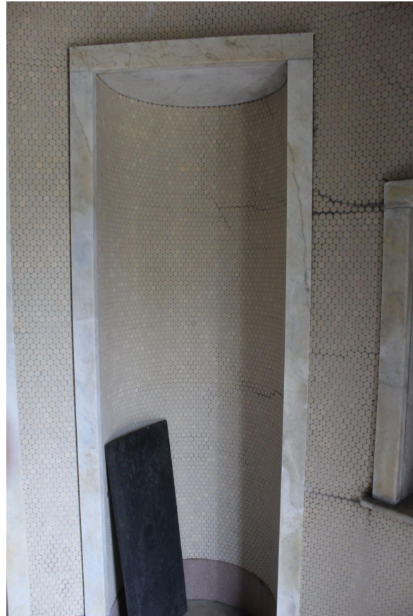
The missing part is leaning in the niche inside - Photo by the author (2.4)
