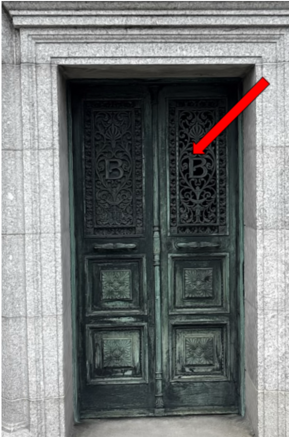
Missing part of the door, where you can see inside - Photo by the author (2.3)
