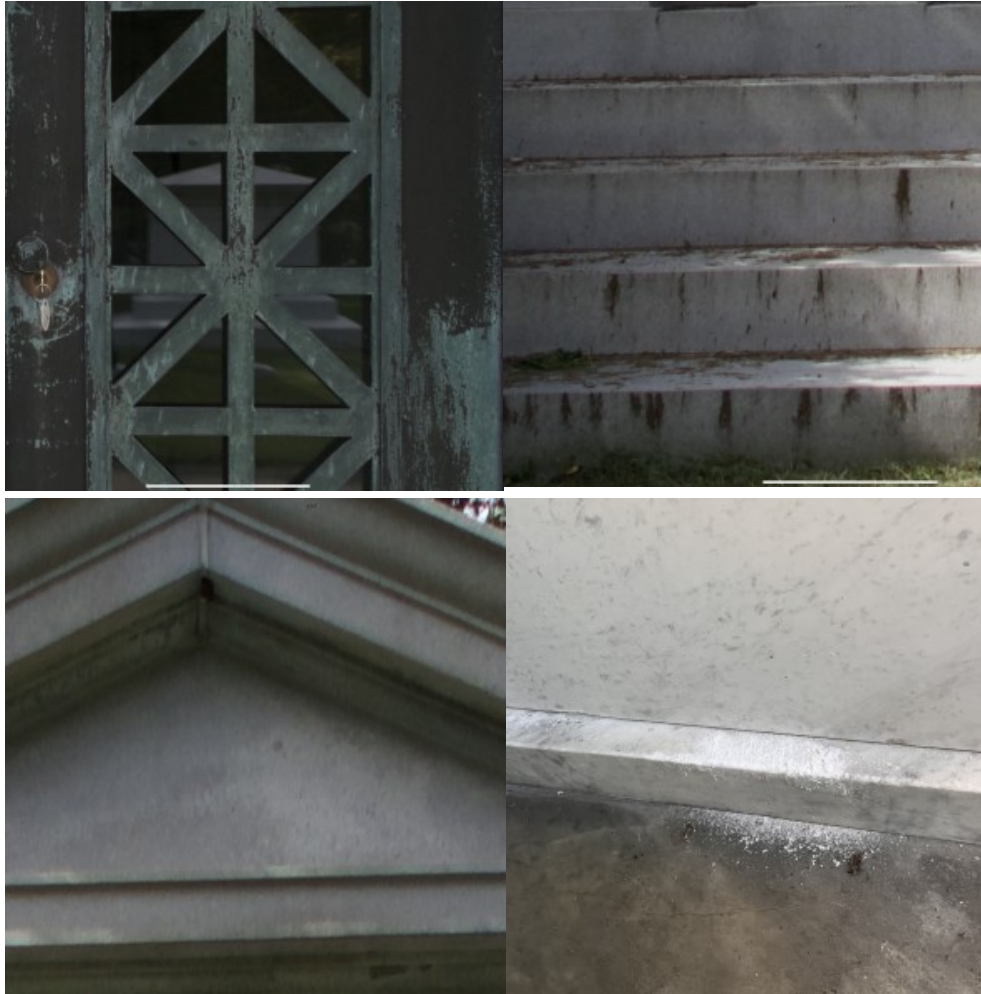
Figure 6: Building Corrosion (Author, 2023)
